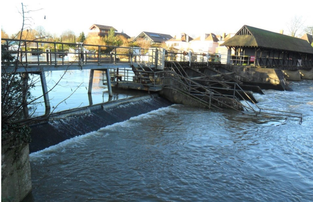
Figure 4-9: Photograph of the existing overfall weir (far left) on weir C at Molesey.
